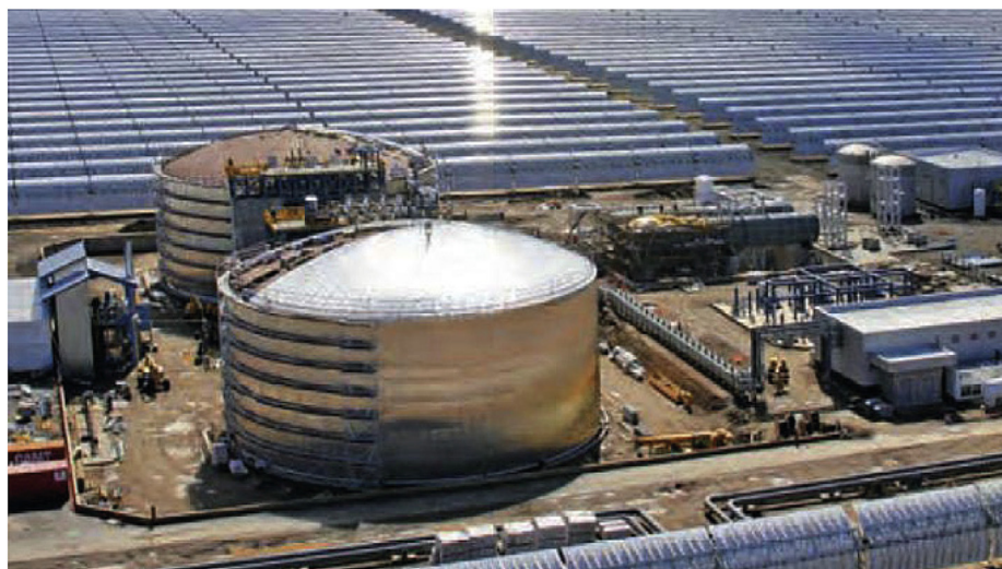
Fig. 4. A molten salt TES pilot plant located in Seville (Spain) [65].
