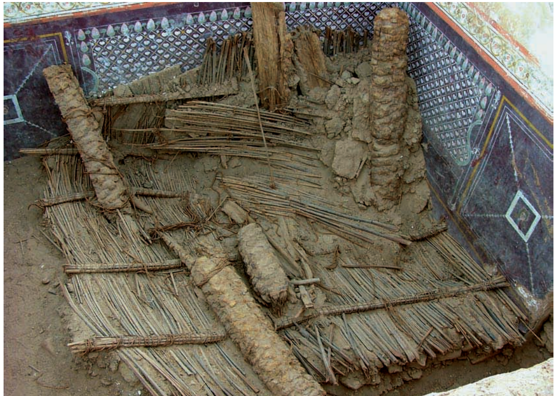
FIGURE 18. Kellis, building B/3/1: collapsed roof and wall paintings in Room 6 (courtesy of C. A. Hope).
