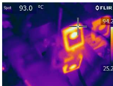
Figure 2-21: Thermal image of the half bridge MOSFET boost side.
