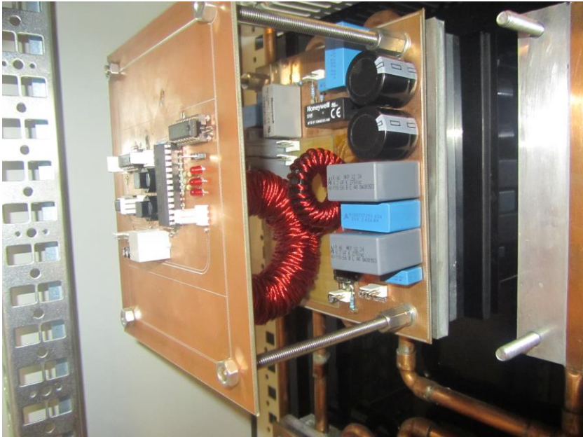
Figure 2-6. Control board of one of the DC-DC converters interfacing the photovoltaic field with the DC bus.
