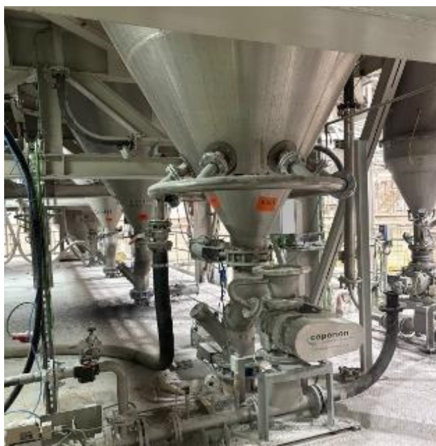
Figure 3. Silo installment: the hot air is introduced through the circular bottom tubes.
