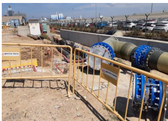
Figure 3.3. Electrical enclosure (back), WWTP feed (left pipe) and WWTP outlet (right pipe).
