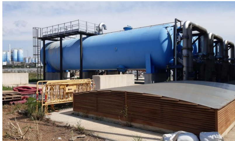
Figure 2.6. Closed sand filters.
