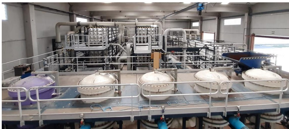
Figure 2.7. Cartridge filters (front) and reverse osmosis racks (back).
