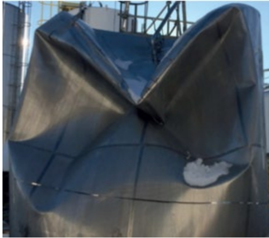
Figure 6: Low-pressure storage tank after its implosion. [10]
