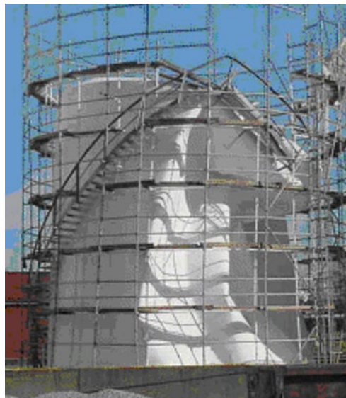
Figure 7: Implosion caused by the obstruction of the outlet orifice. [10]
