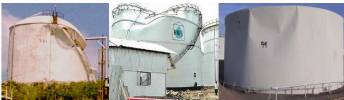
Figure 5: Some examples of tank implosions due to vacuum. [10]
