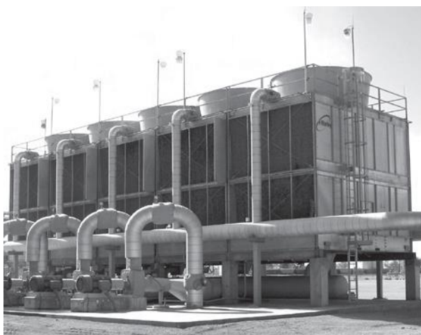
Figure 3.11. Factory-Assembled multicellular cooling tower.
