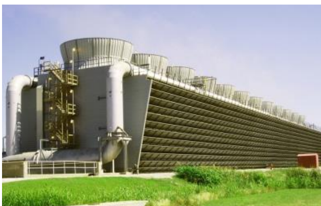
Figure 3.12. Field-Erected multicellular cooling tower.
