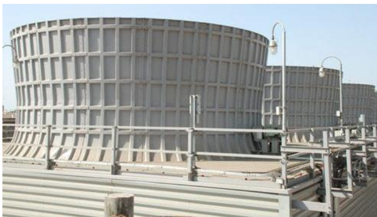
Figure 7.4. Cooling tower fan cylinder.
