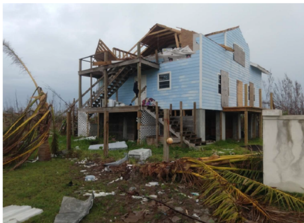
Figure 1.1: A photo taken after Hurricane Dorian in 2019 shows how the walls and roof of a one-story elevated house on Abaco Island were damaged by the storm [4]
