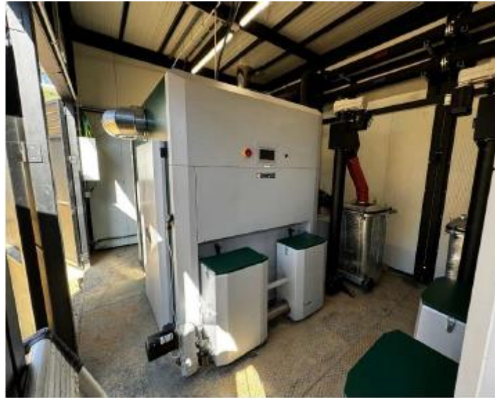
Figure 2.5. Biomass boiler installed in the Córdoba demo site.
