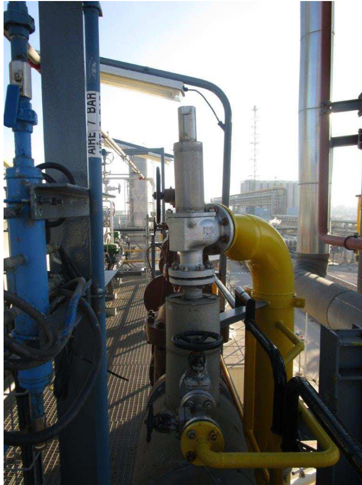
Figure 7.21: Picture of YS861-04 and protected equipment.
