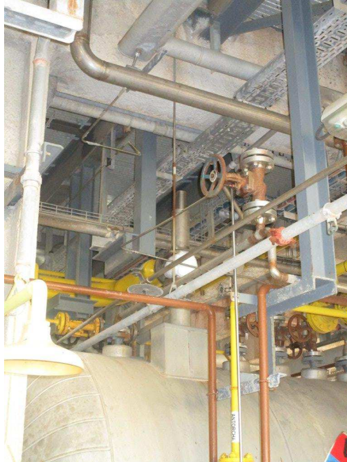
Figure 7.18: Picture of YS860-01 and protected equipment.
