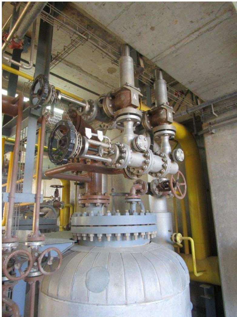
Figure 7.13: Picture of YS701-01/02 and protected equipment.
