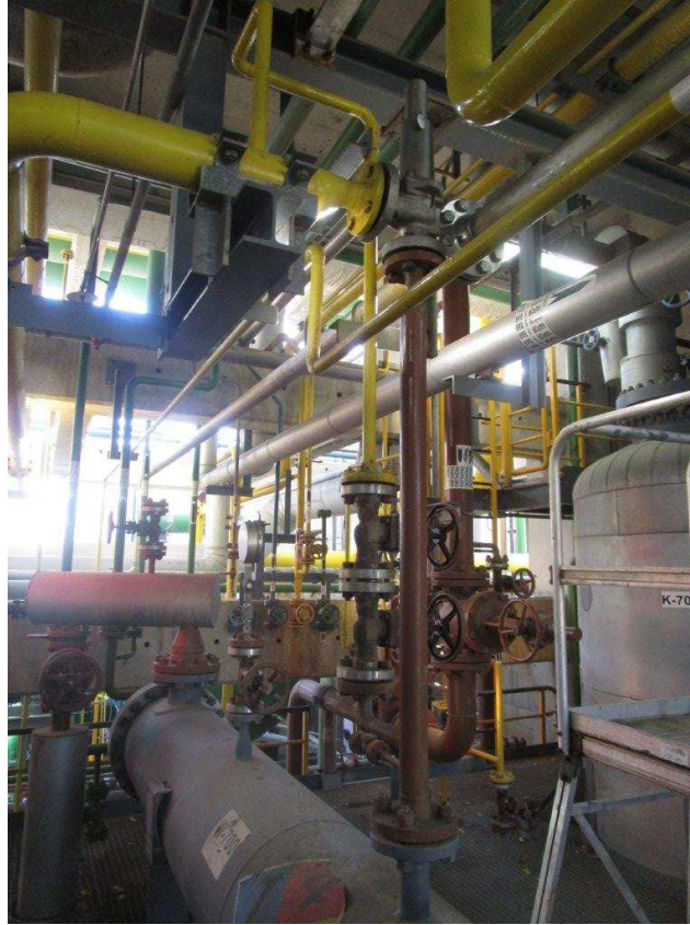
Figure 7.8: Picture of YS702-01 and protected equipment.
