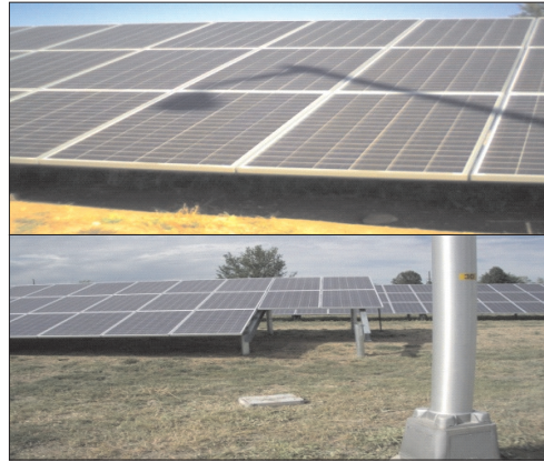
Figure 12. Scenario I: utility-scale system. Top image shows detail of partial shading from nearby light poles.
