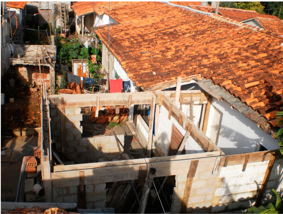
Figure 2. Examples of changes to the heritage in the historical centre of Viñales: a house is extended at the expense of the backyard. Source: authors.
