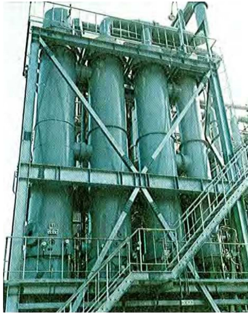
Figure 16: Heat transformer installed 1982: Hitachi Zosen Corp., nominal capacity \approx 1.7 MW [51]
